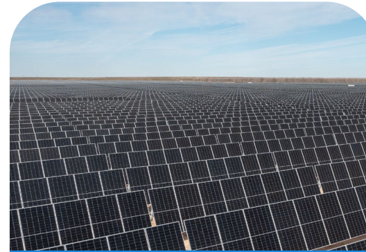
Ashtrom Renewable Energy
